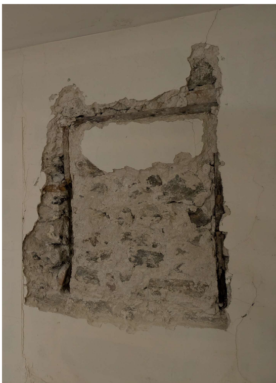
Example of an area of wall plaster removal
