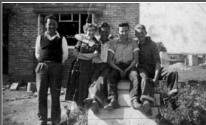
Gerry Thompson working on new houses in Limavady, 1953 © Janis Thompson Bolan collection Coleraine Museum
